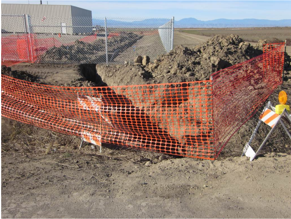
Photo 1: Trench excavation for the 8-inch saltwater connection line between the Remote Well Pad site and the saltwater disposal well.
