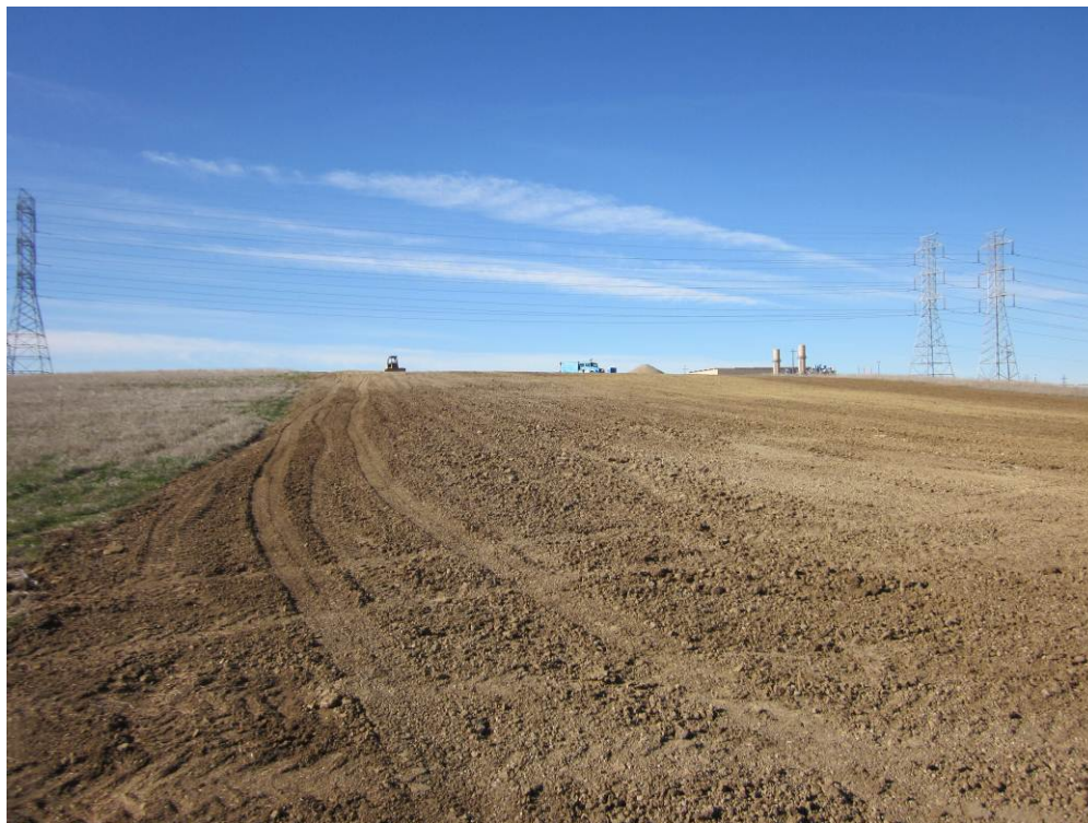
Photo 5: Temporary work area between the 400/401 Line Interconnect and the Metering Station. Pipeline has been buried and backfilled and final grading is underway by PG&E crews.
