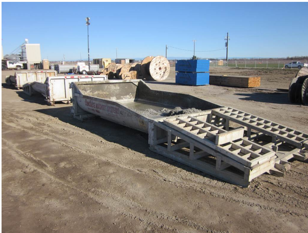
Photo 3: Concrete washout provided at the Compressor Station site for containment of excess concrete.
