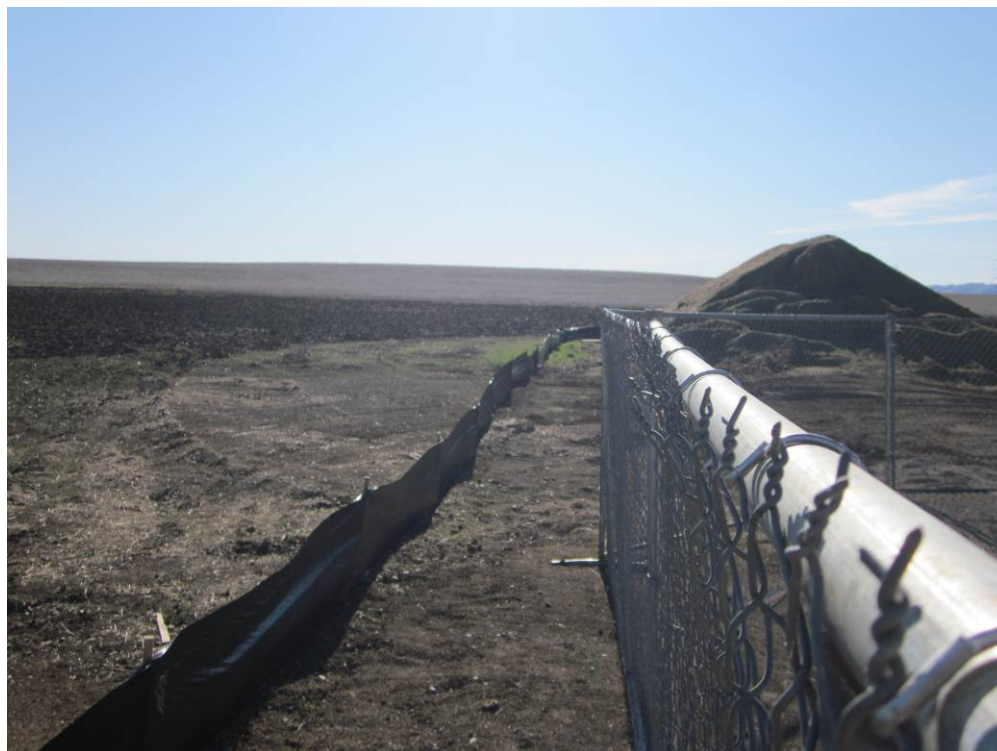
Photo 6: Intact silt fence and hydroseeded soil stockpiles at the Metering Station where it connects to the 25-inch natural gas pipeline.
